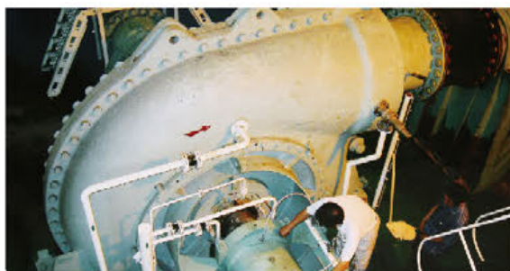
中交天津航道局800WN泵运行检查 CCCC Tianjin Dredging Co., Ltd., 800WN Pump Operation Inspection
