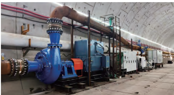
上海基础设施建设15米300SGH 泵站运行 Shanghai Infrastructure 15m 300SGH Pump Station Operation
