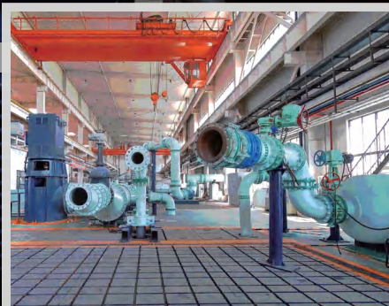
High-Voltage Pump Test Station
